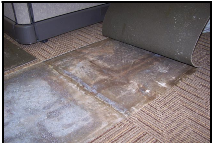
SLAB MOISTURE UNDER CARPET TILES
