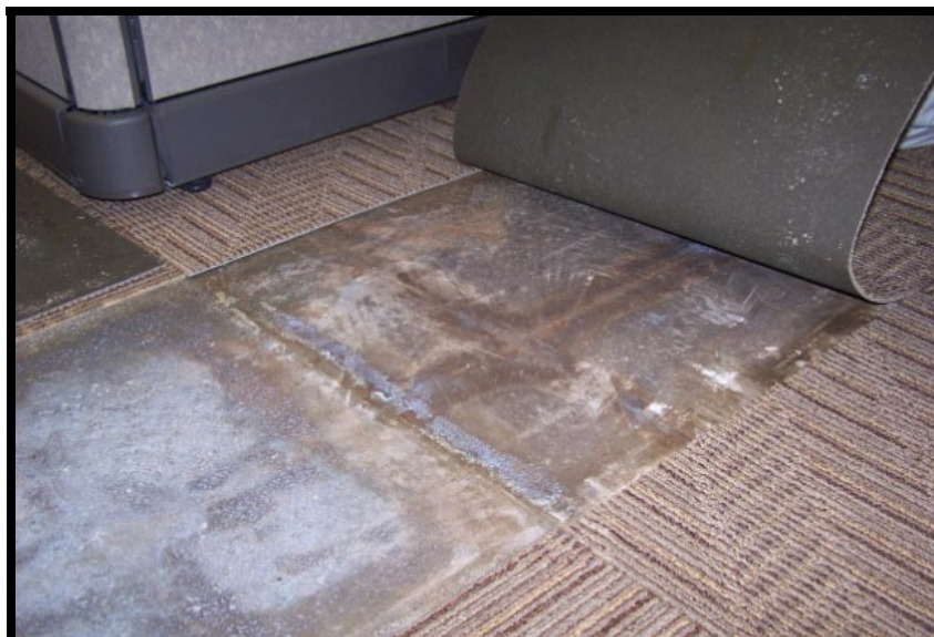
SLAB MOISTURE UNDER CARPET TILES
