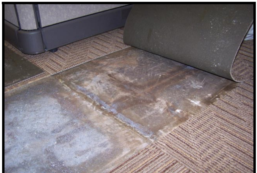
SLAB MOISTURE UNDER CARPET TILES
