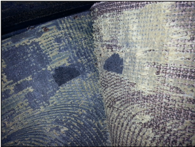
Failed Double Stick Installation
