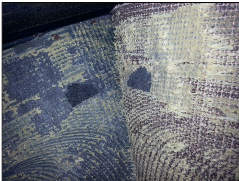
Failed Double Stick Installation
