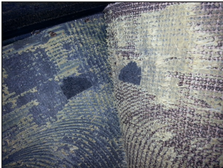
Failed Double Stick Installation
