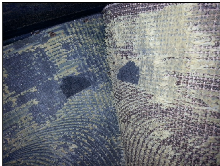
Failed Double Stick Installation
