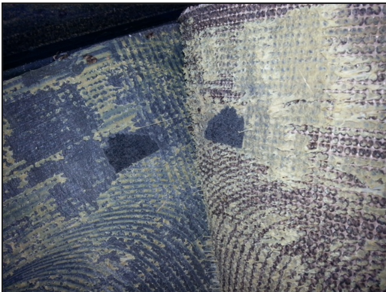
Failed Double Stick Installation
