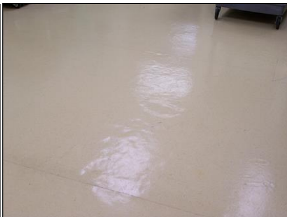
Poor Floor Prep
