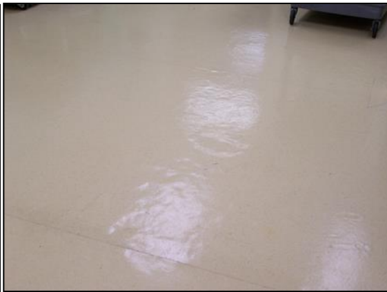
Poor Floor Prep
