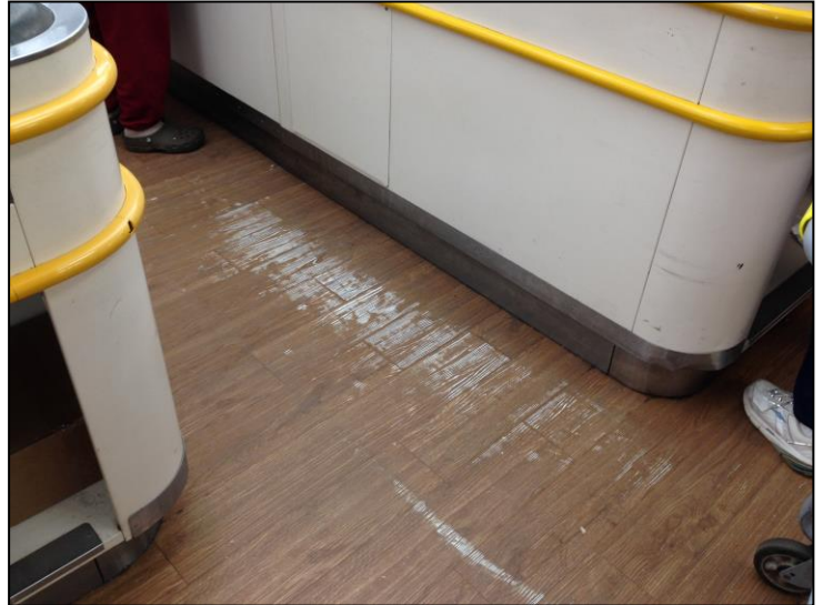
LVP Finish Loss from Traffic
