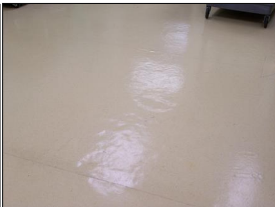
Poor Floor Prep
