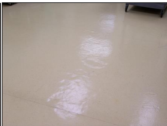
Poor Floor Prep
