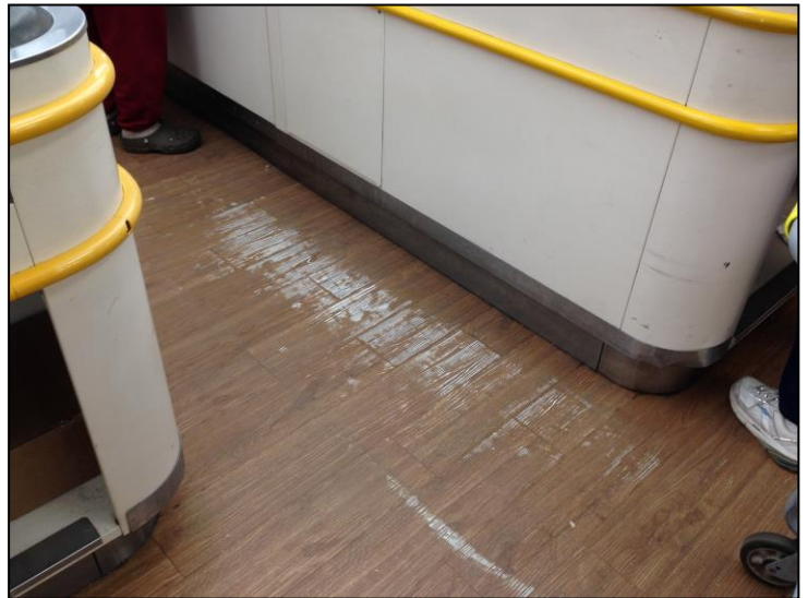
LVP Finish Loss from Traffic
