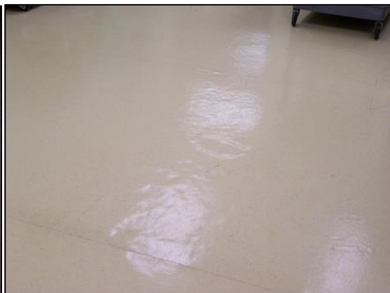
Poor Floor Prep
