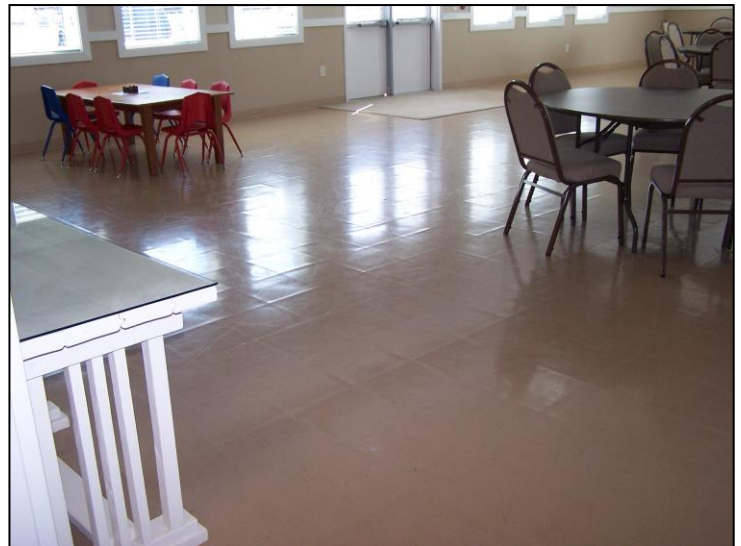
VCT Tile Water Damage
