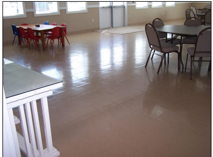
VCT Tile Water Damage
