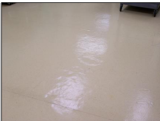
Poor Floor Prep
