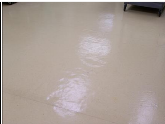
Poor Floor Prep
